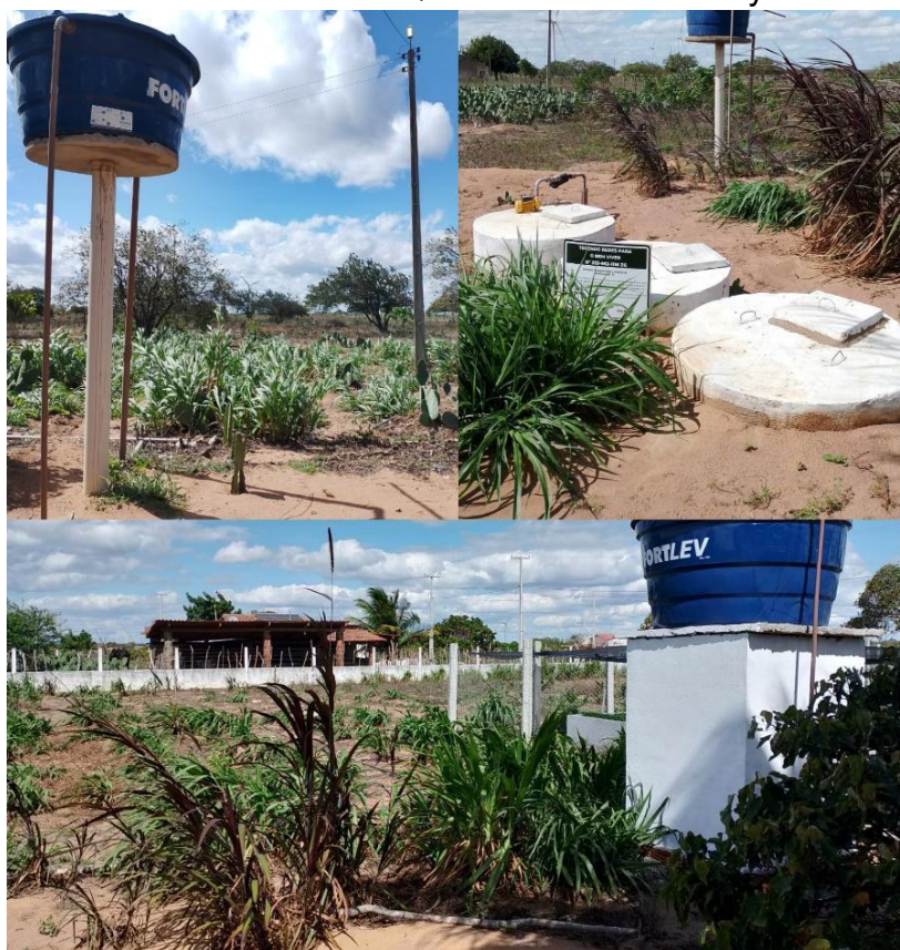
Figure 02 – Bioágua greywater reuse system installed by the Diocesan Caritas of Caicó in the Macambira Quilombola Community
